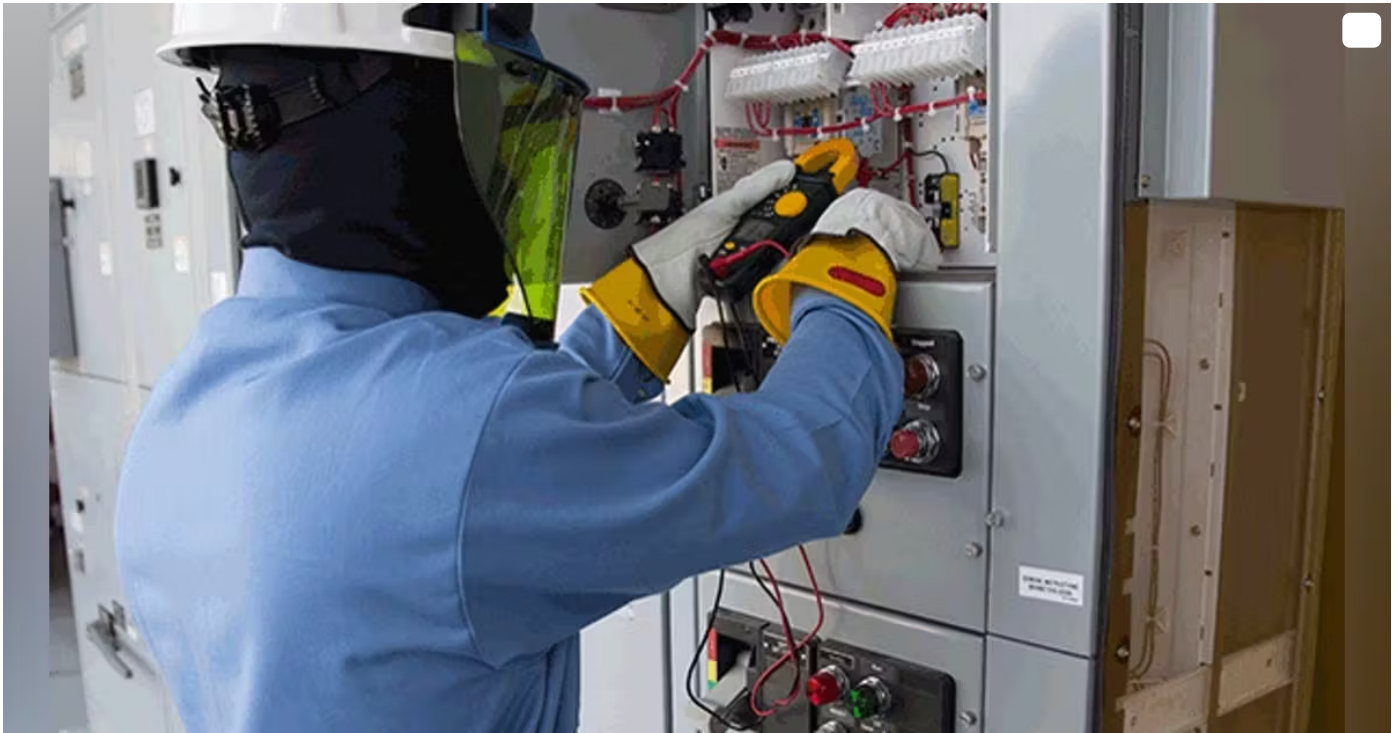
An electrical worker is geared up in arc flash workwear, which includes rubber insulated safety gloves, a hard hat, and face shield.
